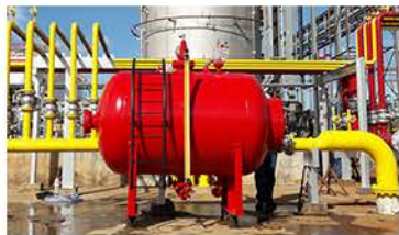
Foam Tank & Foam Equipment
